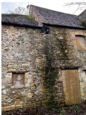
West elevation with missing downpipe and misaligned hopper
